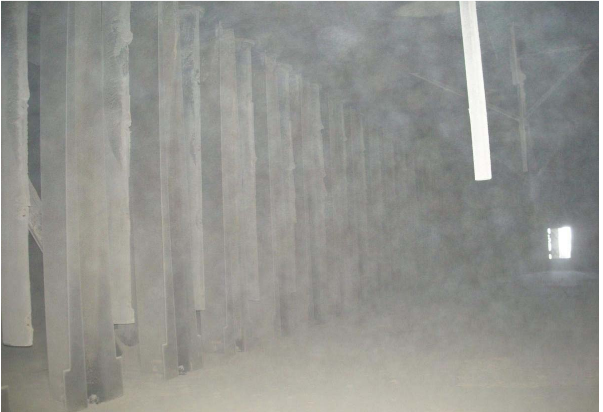
Injection Duct – Fall 2010; after 8 months of operation
